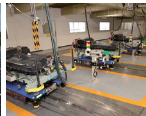
MX-30 EV battery charging stations
