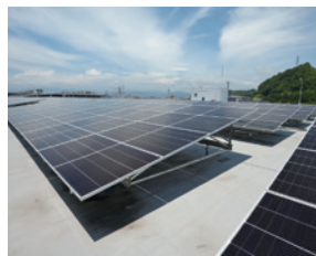
Hiroshima Plant's rooftop solar panels
