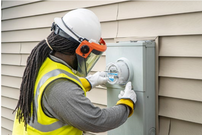
Smart meters like this one can be turned on and off remotely, permitting faster service and reducing service vehicle emissions.
