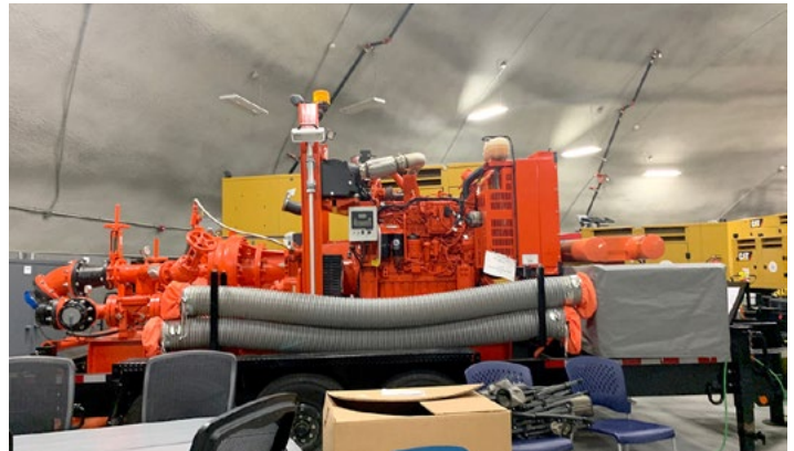
A Godwin pump, used to provide water to key systems, sits in a storage dome where backup equipment is kept at our Surry Power Station in Virginia.
