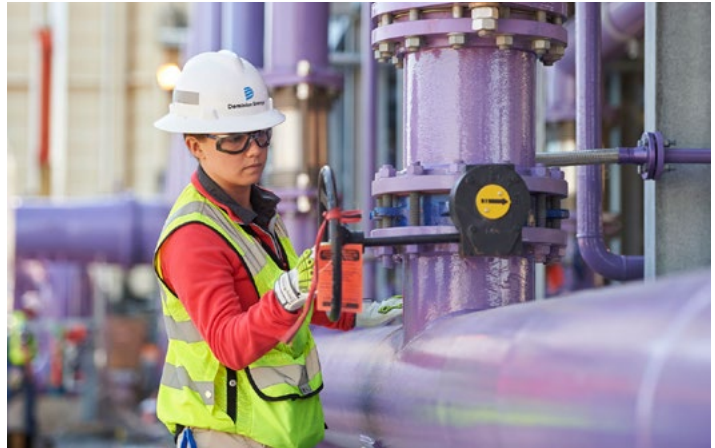
Workers at the Brunswick County Power Station produce electricity from clean natural gas, powering 340,000 homes and businesses.
