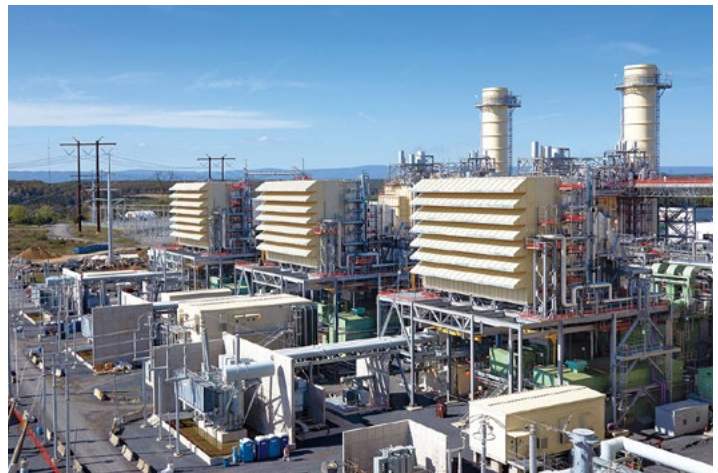
Warren County Power Station.
